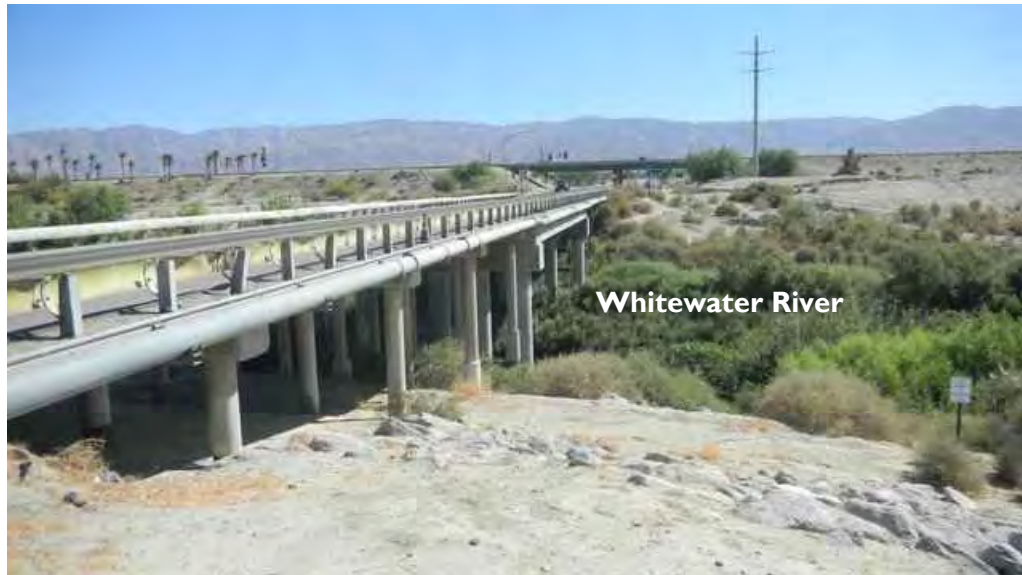
Figure 3-4: Bridge Crossing the Coachella Valley Stormwater Channel (Whitewater River) at Dillon Road
