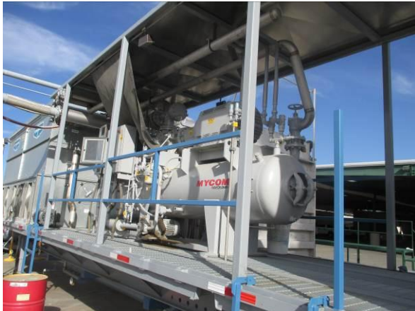
Photo #25 View of Ammonia AST associated with the Hydrovac unit.
