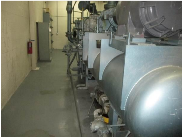
Photo #37 Typical view of engine room B.
