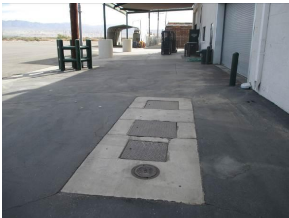
Photo #41 View of oil/water separator adjacent to the north of the building.
