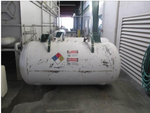
Photo #31 View of Ammonia ASTs associated with the cooling system to the east of the building.
