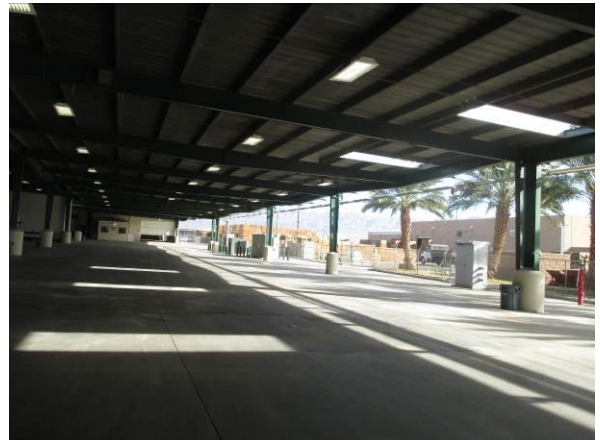
Photo #2 View of receiving canopy located to the southeast of the site building.
