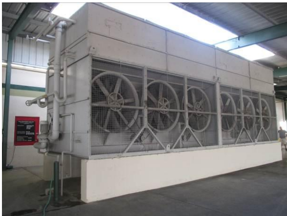
Photo #33 View of air cooling machine located on the central portion of the northern parcel.
