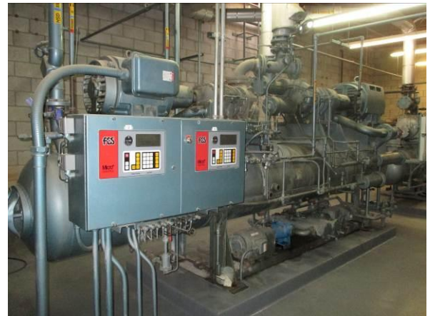
Photo #28 View of engine room A located in the central portion of the building.
