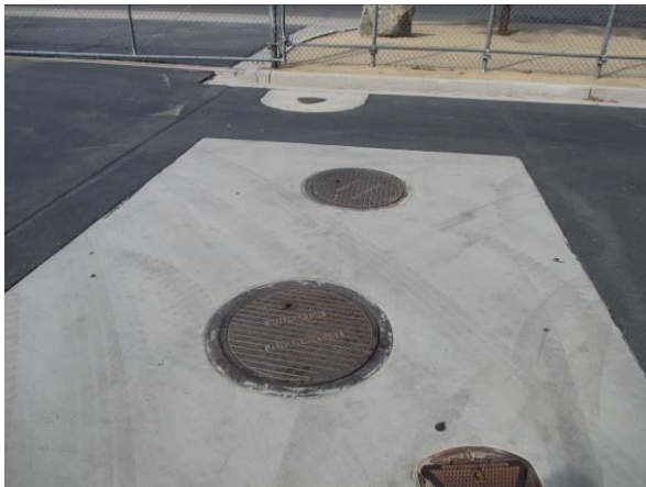
Photo #51 View of interceptor located on the southwestern portion on the northern portion of the northern parcel.
