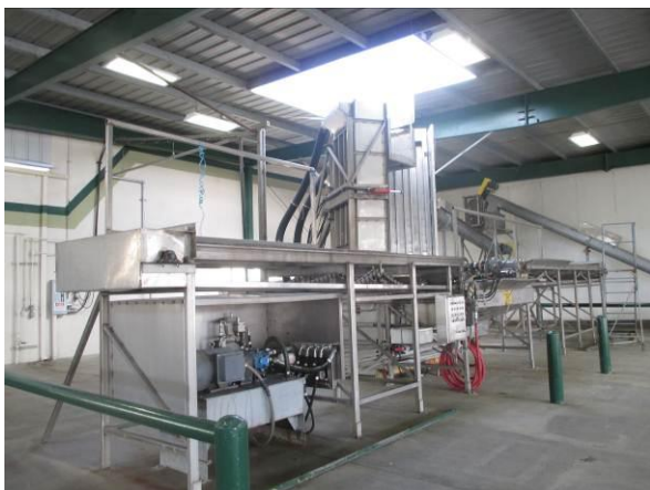
Photo #35 View of ice crusher machine on the central portion of the northern parcel.
