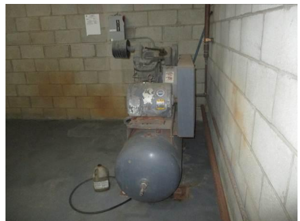
Photo #30 View of air compressor within engine room A.
