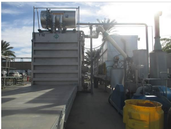
Photo #23 View of the Hydrovac unit on the southern portion of the northern parcel.
