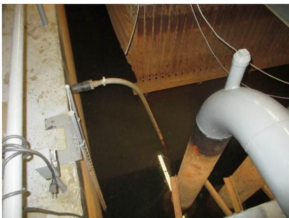
Photo #29 View of open concrete pit associated with the engine room A.
