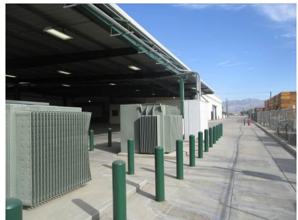
Photo #36 View of pad-mounted transformer on the eastern portion of the northern parcel.
