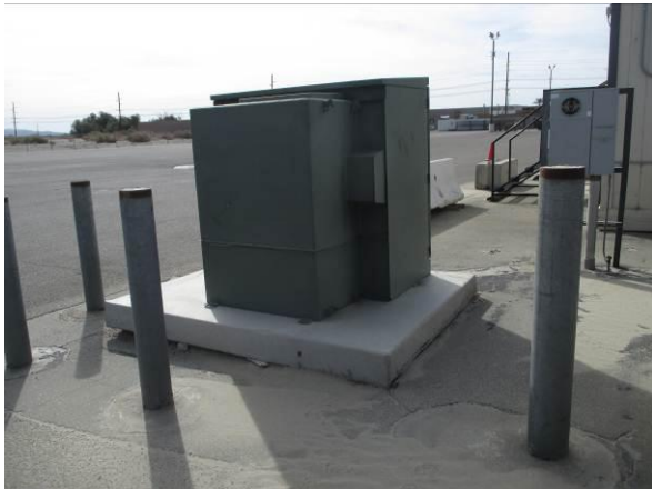
Photo #49 View of pad-mounted transformer located on the northeastern portion on the northern portion of the northern parcel.
