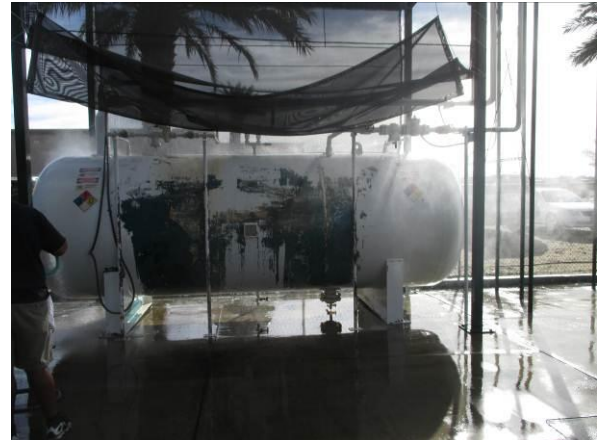
Photo #26 View of the 1,000-gallon propane AST on the southeastern portion of the northern parcel.
