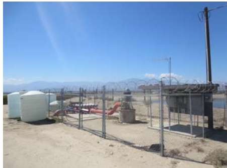
GROUNDWATER WELL, ASTS, AND TOTE EAST OF WATER RETENTION POND, LOOKING SOUTHWEST
