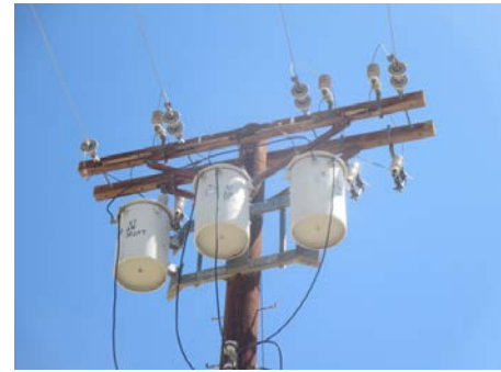
POLE MOUNTED TRANSFORMERS NEAR THE WATER RETENTION POND, TYPICAL OF THREE ON THE PROPERTY
