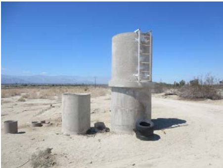
UTILITY ACCESS PIPES FOR WATER AND SEWER, BY THE WATER RETENTION POND, LOOKING WEST, TYPICAL OF MANY THROUGHOUT THE PROPERTY
