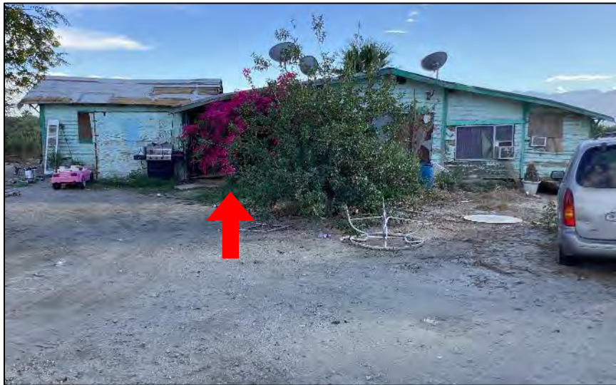
Photograph 8: North elevation of Building A. The location of the front porch is marked with the red arrow. Camera facing south, October 6, 2022.
