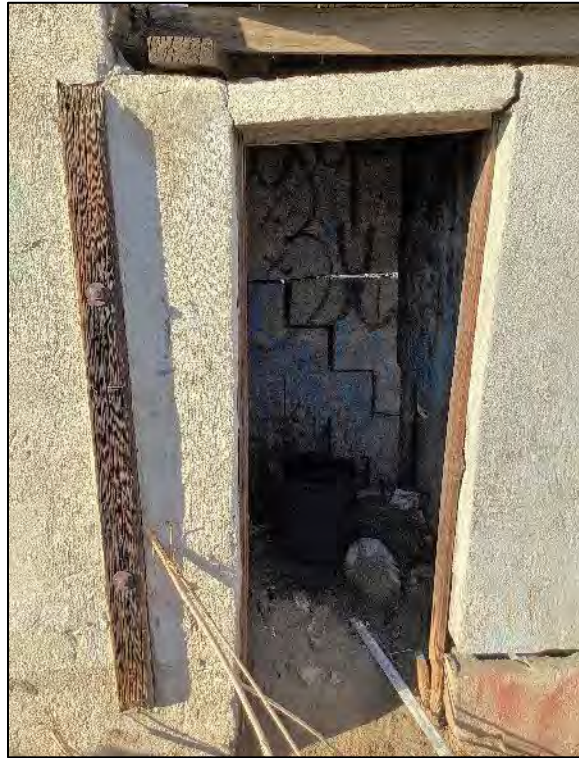
Photograph 16: Entrance to Building B, located on the south side. Camera facing north, October 6, 2022.
