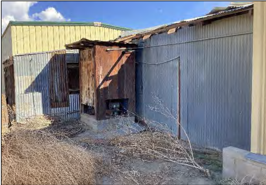
Photograph 21: Angled view of the north side of Building D, showing the depth of the one-room extension at the northeast corner and the utility enclosure. Camera facing southeast, October 6, 2022.
