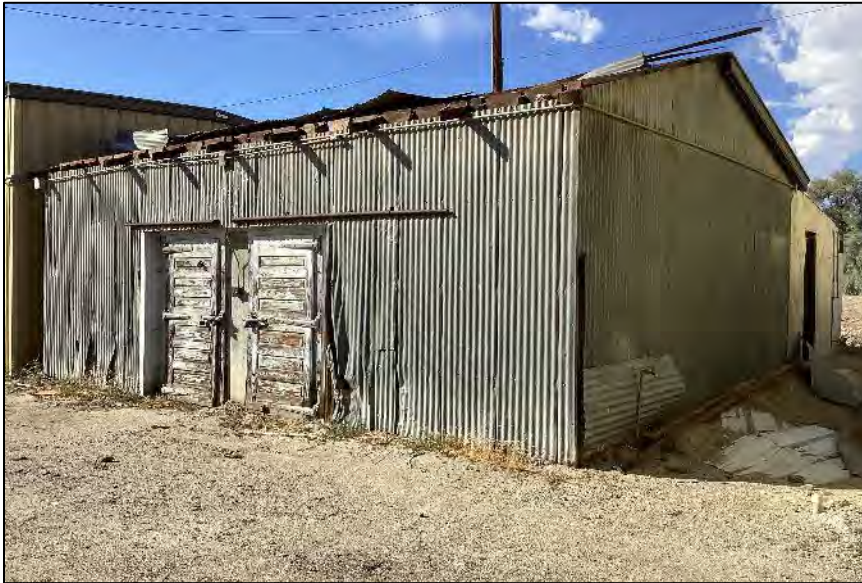
Photograph 19: Primary south side and east gable end of Building D. Camera facing northwest, October 6, 2022.
