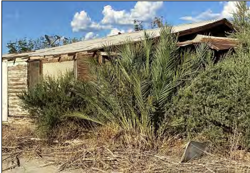
Photograph 10: Rear, south side of Building A viewed from the southwest corner. Note the location of the rear porch (right). Camera facing northeast, October 6, 2022.
