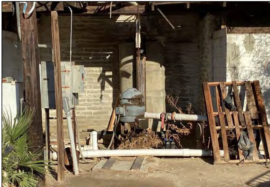
Photograph 3: Irrigation pump, sheltered under Building E. Camera facing east, October 6, 2022.
