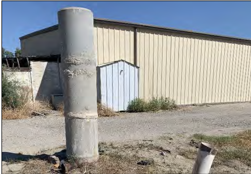
Photograph 6: Exposed concrete pipe located south of Building E (left) and Building J (right). Camera facing northeast, October 6, 2022.
