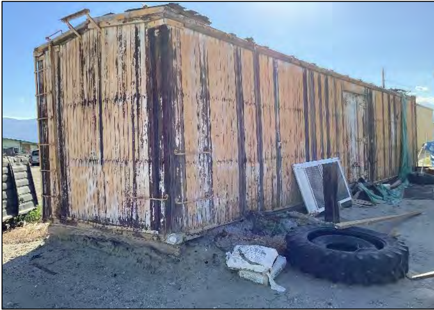
Photograph 25: East end and north side of the box car. Camera facing southeast, October 6, 2022.
