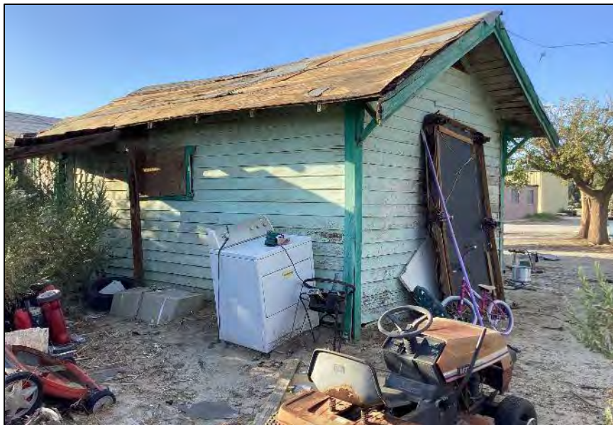
Photograph 11: Gabled addition located at the southeast corner of Building A. Camera facing northwest, October 6, 2022.
