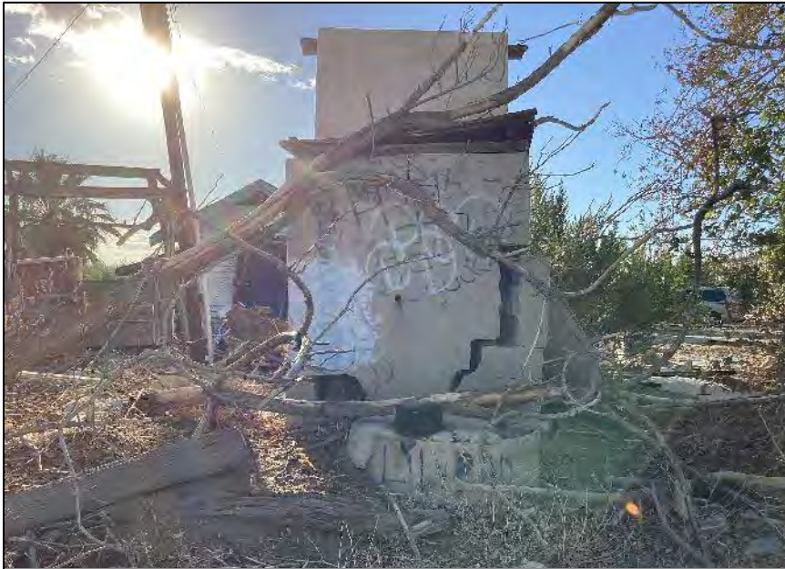
Photograph 14: East end of Building B, showing large crack in the wall. Camera facing west, October 6, 2022.
