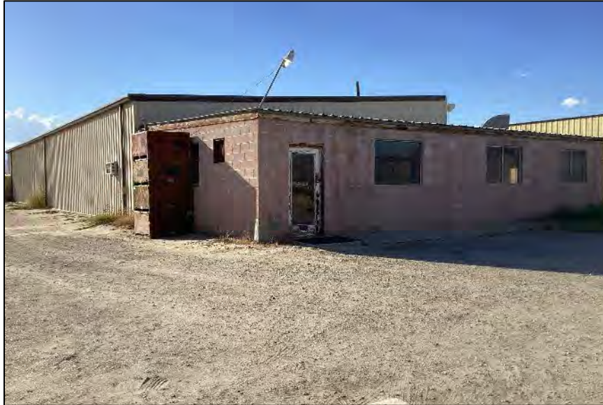
Photograph 17: South end and east side of Building C, showing main entrance at the southeast corner. Camera facing northwest, October 6, 2022.
