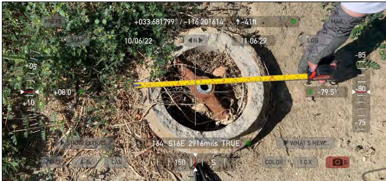
Photograph 7: Exposed irrigation valve located south of Building J. Additional concrete piping above the valve appears to have been removed. October 6, 2022.
