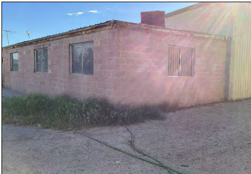
Photograph 18: East side and north end of Building C. Camera facing southwest, October 6, 2022.
