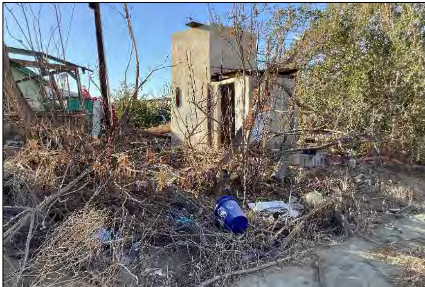
Photograph 13: Contextual view of Building B, viewed from the southeast corner. Camera facing northwest, October 6, 2022.
